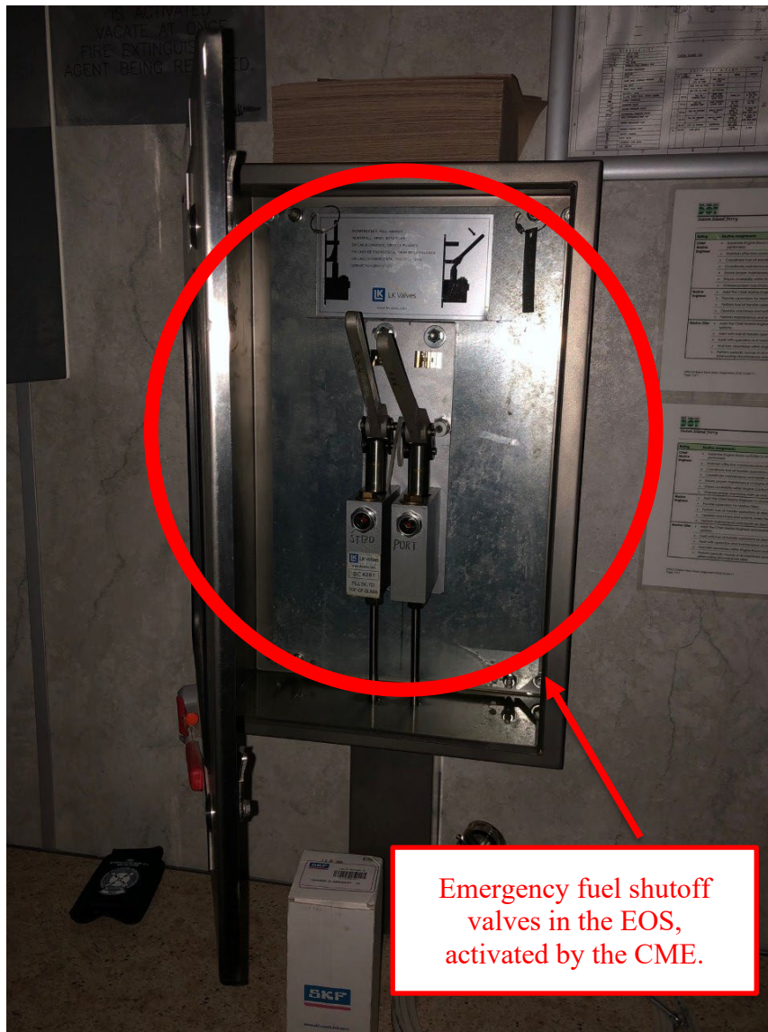
Figure 9. Photograph of the emergency fuel shutoff valves located in the EOS taken on December 27, 2022. Provided by the U.S. Coast Guard.
