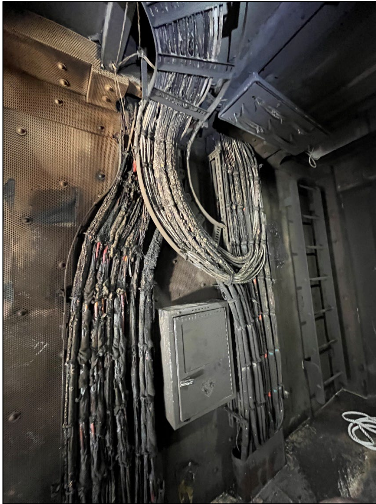
Figure 14. Photograph of damaged cables located in the main deck machinery casing above the engine room. Provided by the NTSB.
