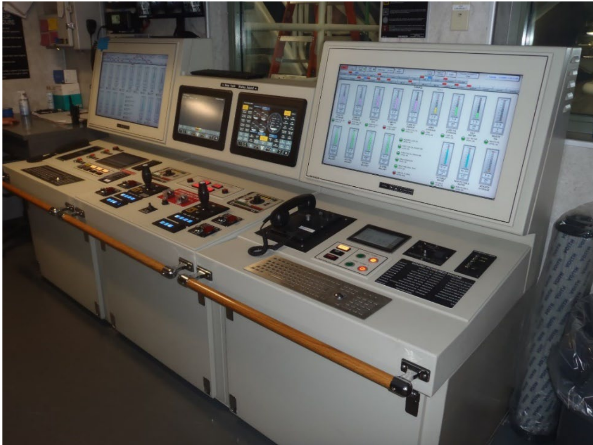
Figure 2. Photograph of the Machinery Control Station (MCS) in the Engine Operating Station (EOS) with the tank level indication display onboard the SANDY GROUND's sister vessel, the SSG MICHAEL H OLLIS, taken on December 23, 2022. Provided by the U.S. Coast Guard.
