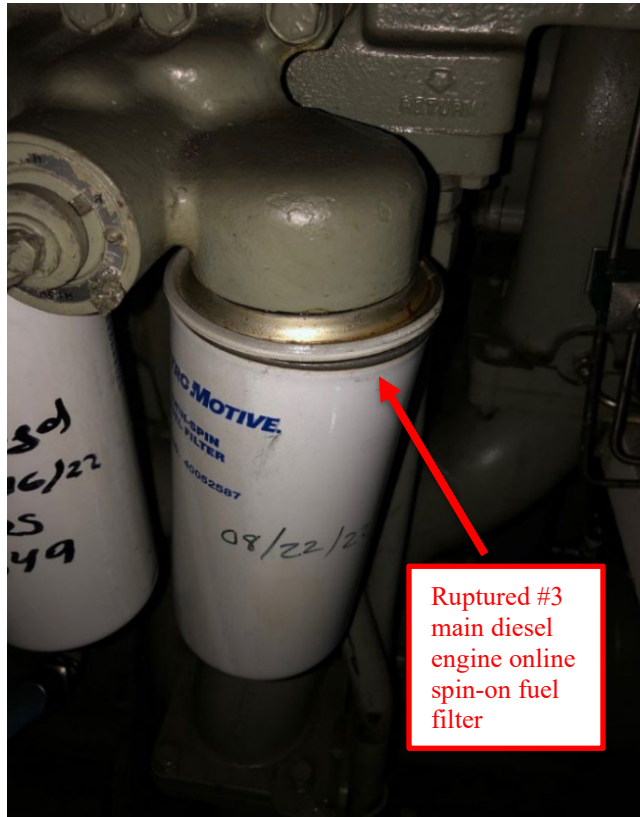
Figure 12. Photograph of the ruptured fuel oil filter on the #3 main diesel engine taken on December 23, 2022. Provided by the U.S. Coast Guard.
